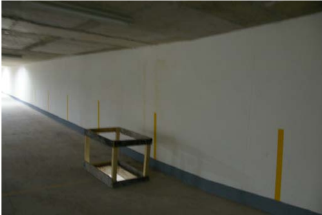
Figure 2 Level -9 Basement Wall of Echeverria Izquierdo Building in Santiago, Chile after February 27, 2010 earthquake
